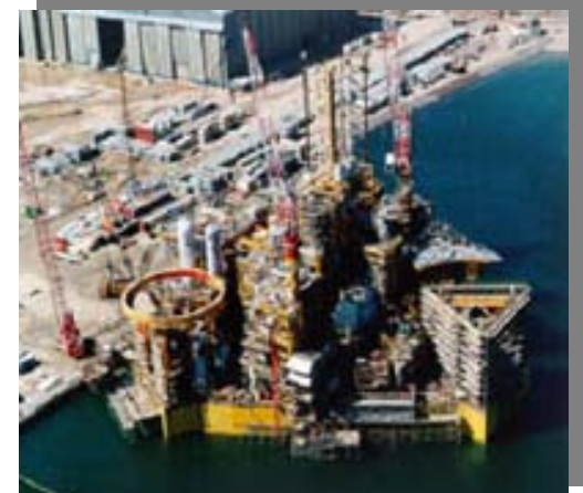
Hook-up & com quay side
